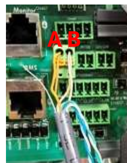
Monteret i inverter
