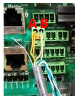
Monteret i inverter
